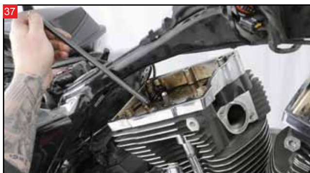
The pushrods and tubes are removed next. Repeat the process for the second cylinder, ensuring it is at TDC of the compression stroke when performing work.
